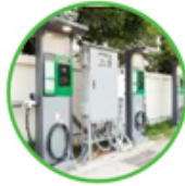
EV Charging Station
